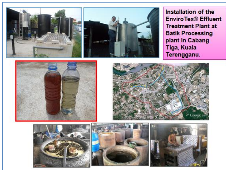
Installation of EnviroTex® Effluent Bio-Treatment for Azo-Dye Waste Water Treatment at Source
