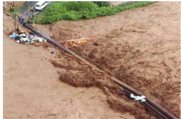
Fig. 5 Flood situation of the RB1 at 11:24 (source Fukui Newspaper)
